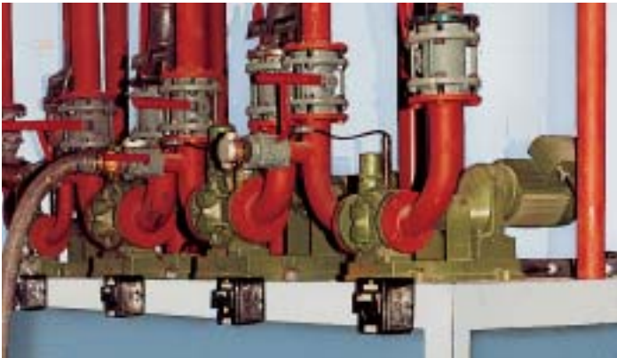
Gear pump TF-GKGM in tank store for binding agents
